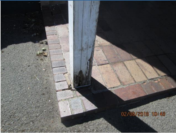
Repaired and eroding post
