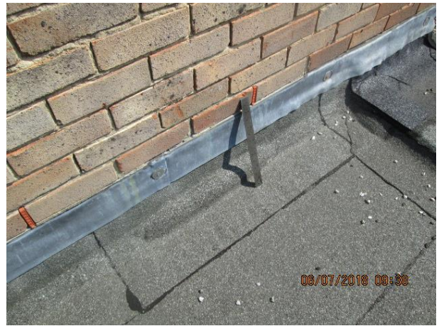
Small felt roof 1 - blister
