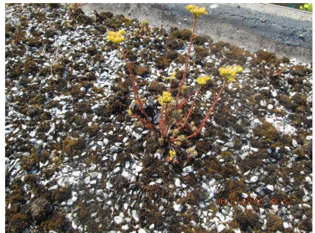
Plant growing in stones and debris on roof
