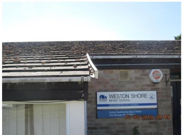
Pitched roof 1 – trim pulling away
