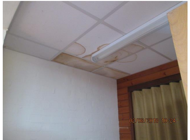
Stained ceiling below pitched roof 1
