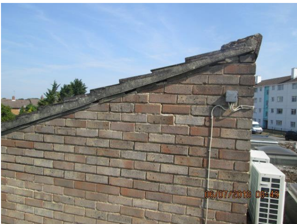
Example of non-roofing fabric requiring repairs
