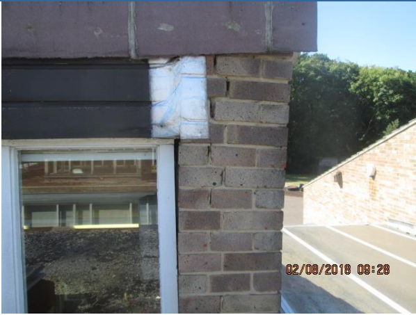
Pitched roof 5 – leaning brick gable and opened joints
