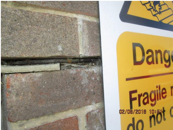
Rusting lintol lifting brickwork
