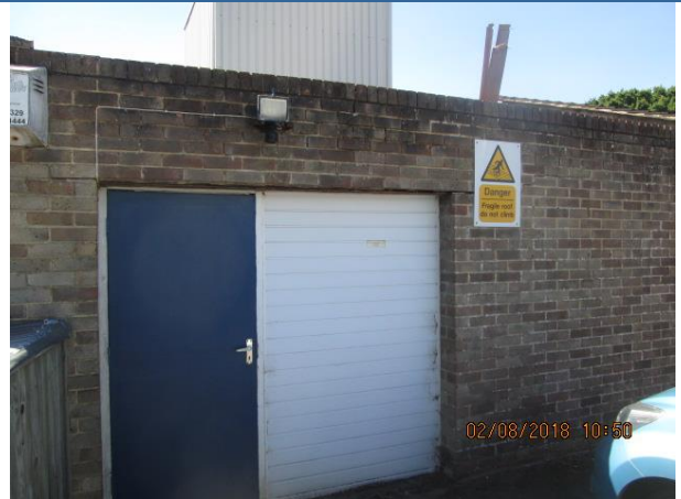
Lintol rusting and lifting brickwork over store door
