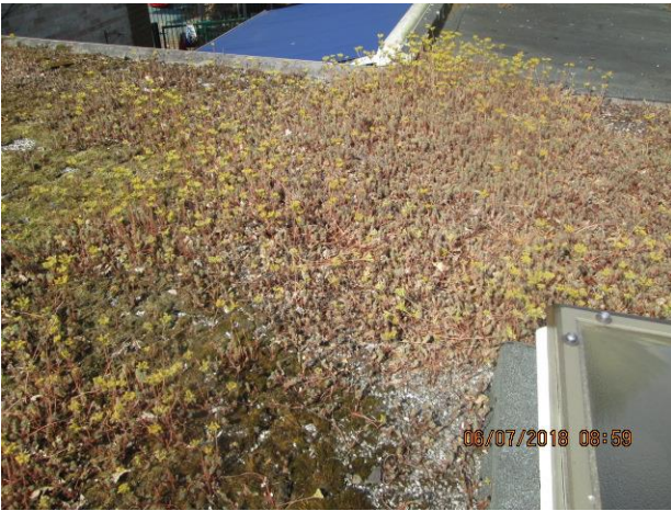
Main roof – Excessive plant growth
