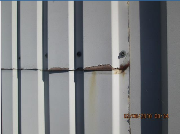
Corroding Tank room cladding at sheet ends
