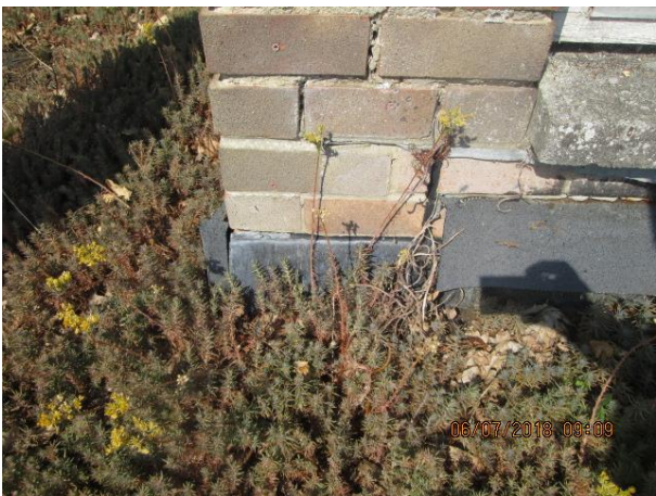
Brickwork cracking and excessive plant growth on roof
