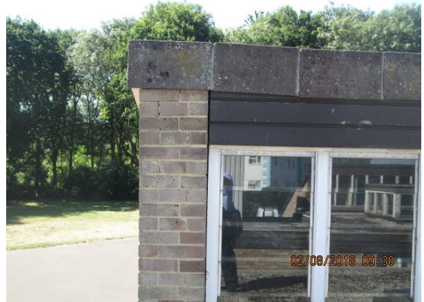
Pitched roof 5 – ridge dropped away from brick wall gable
