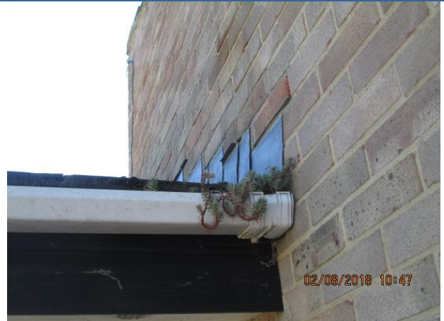
Gutter with plant growth
