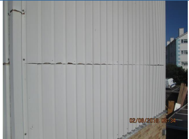
Bulge in cladding - East elevation
