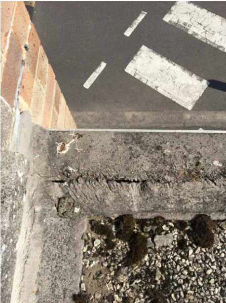
There are splits and cracks in the asphalt. This school was built in 1974 and this is probably the original roof.
