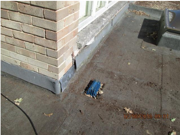
Felt roof 2 swept off exposing felt and gully
