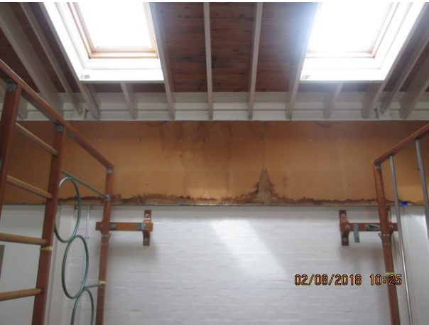
Water staining in hall
