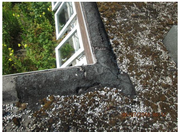
Edge detail patch repair
