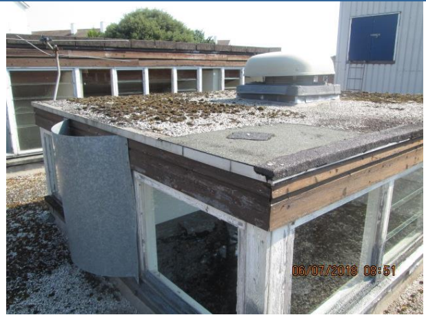
Raised kitchen roof – asphalt with patch repairs
