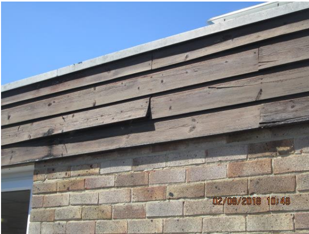
Example of warped and cracking fascia with minimal decoration
