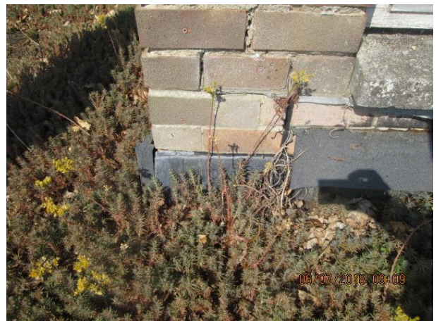
Plant growth and cracking to brickwork, pitched roof 2
