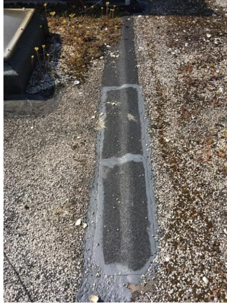
Many areas of this roof have been repaired using either Aquapol or a commodity membrane.
