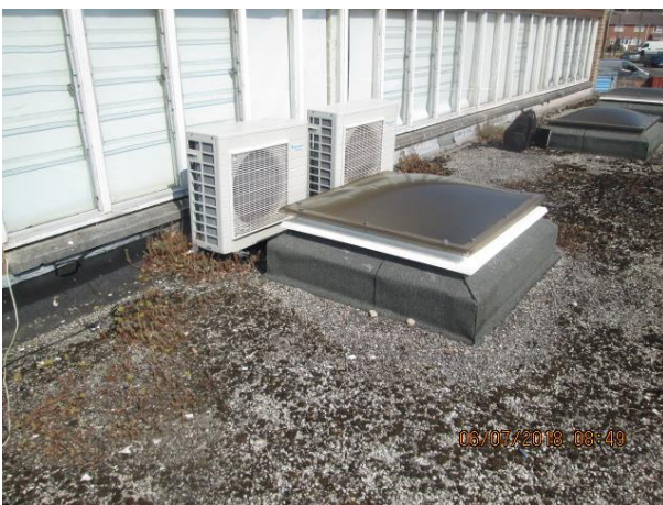
Main roof – Rooflight and Air conditioning condenser on asphalt roof adjacent to pitched roof 3
