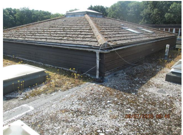
Hall roof above main asphalt roof – one of two downpipes
