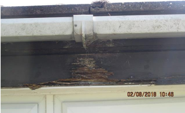
Leaking gutter water damage to fascia
