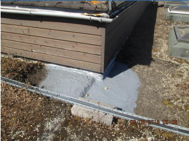
Recent Acrypol repair to asphalt roof adjacent to hall roof North East corner
