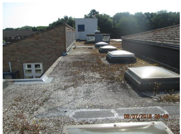
Main roof looking towards tank room, pitch roof 1 on left, hall roof on right
