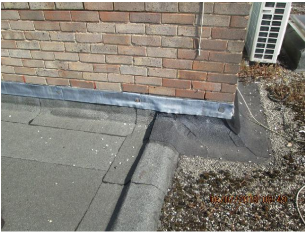
Small felt roof 1 – upstand, flashings screw fixed and blister
