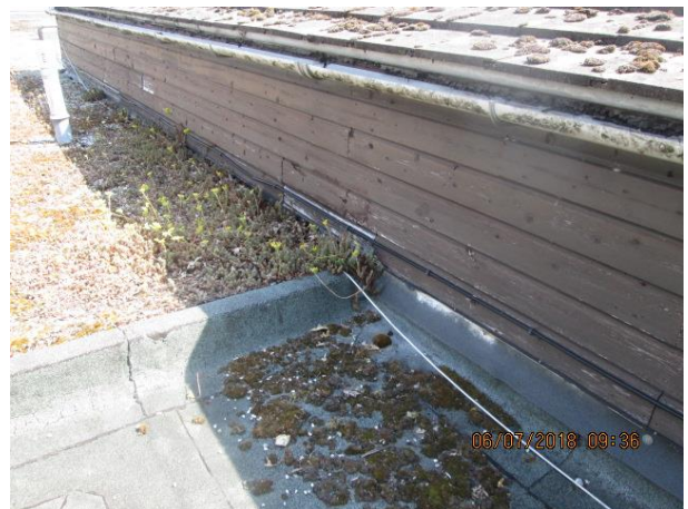
Small felt roof 2 to lower level showing step down from main roof
