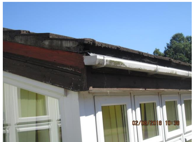
Pitched roof 5 – raised tiles and infill barge board strip
