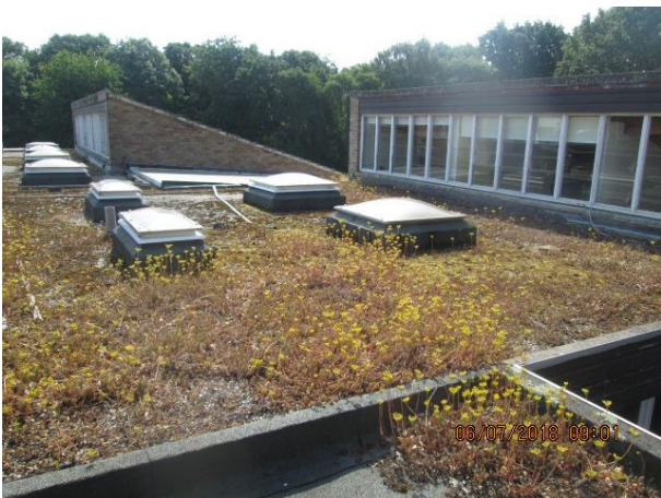
Main roof – plant growth. Pitched roof 4 on right and pitched roof 5 on left
