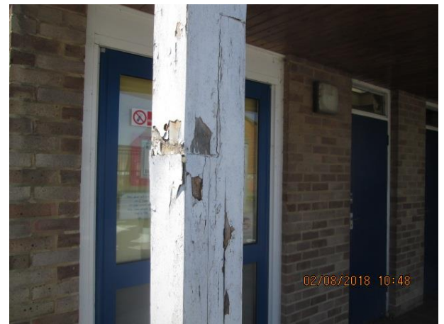
Previous repair to post now failing
