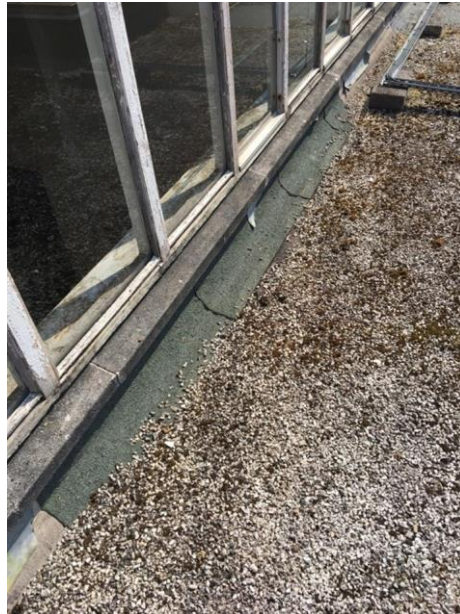
The area under the windows shows where the cover flashing is missing and a repair using felt has been carried out.
