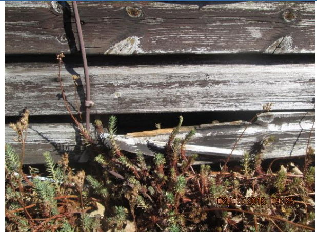
Broken hall roof cladding and plant growth below
