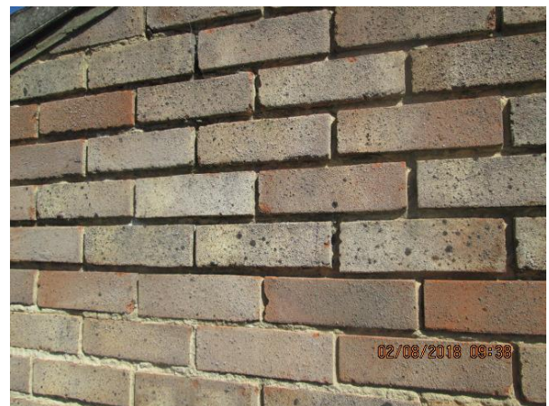
Pitched roof 2 – eroded pointing
