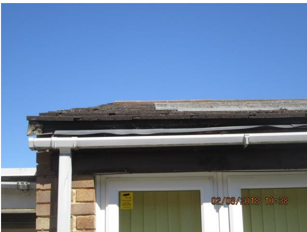
Pitched roof 5 – raised tiles but gutter at original lower level
