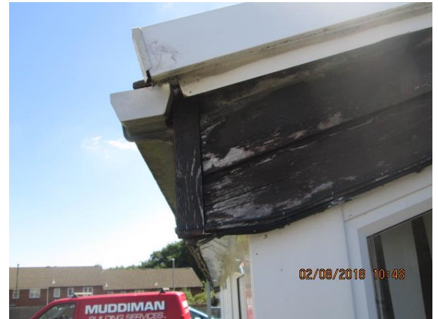
Degraded timber barge board
