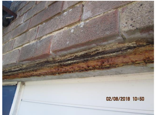
Rusting lintol over store door
