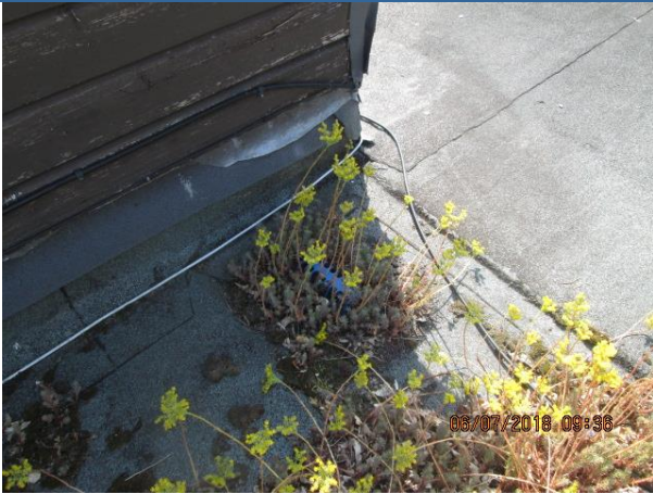
Small felt roof 2 – plants and debris in gully
