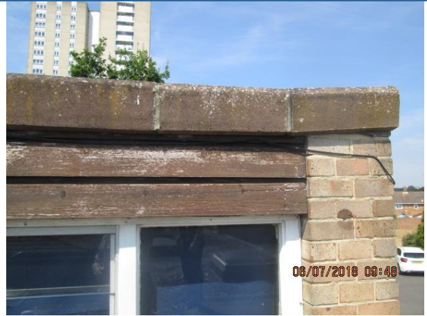
Area of building requiring maintenance
