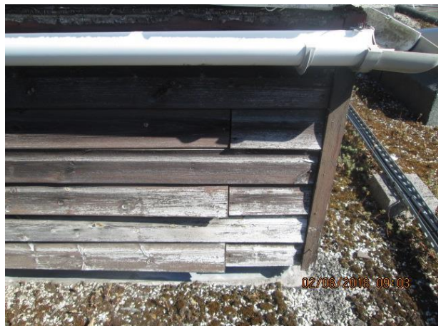
Warped and cracked cladding
