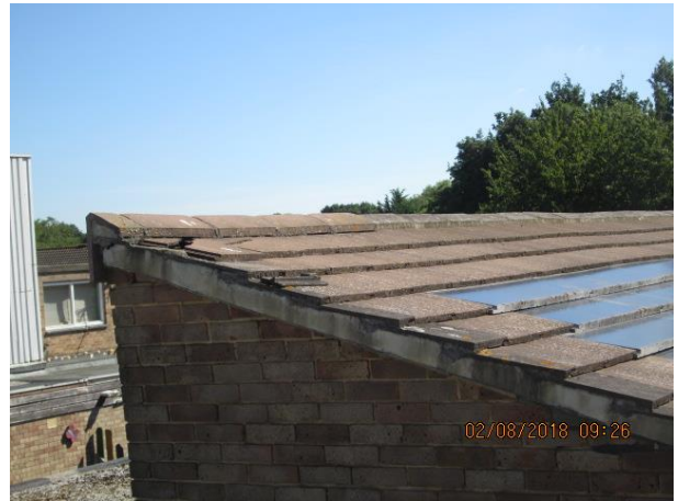
Pitched roof 5 – broken tiles
