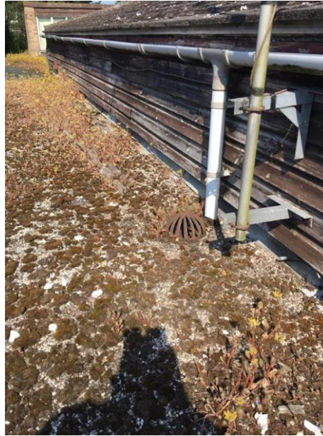
More evidence of ponding water.
