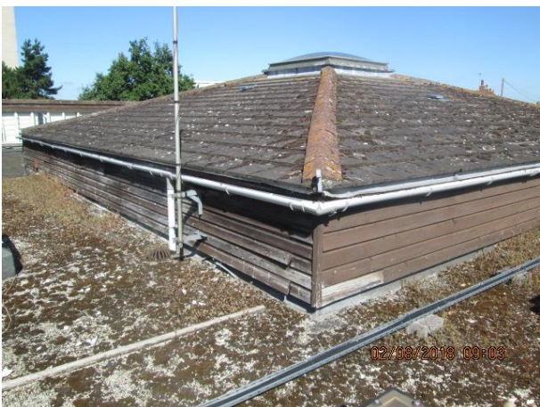
Hall roof. Decaying cladding and poor guttering
