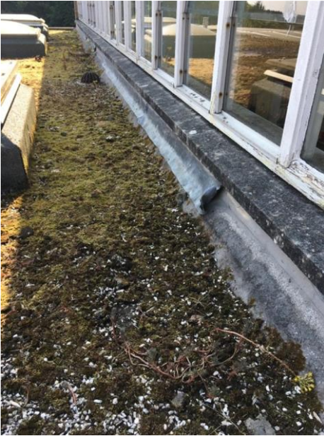
The amount of vegetation on the roof suggests that ponding water is a real issue.
