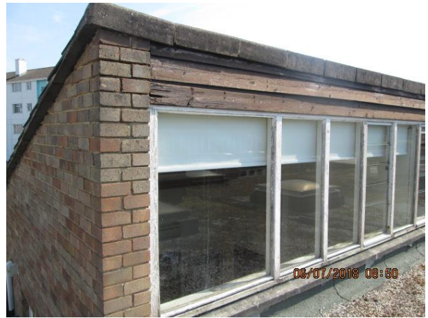
Area of building requiring maintenance and single glazing
