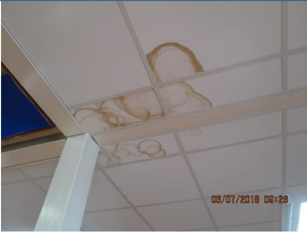
Water staining to corner of hall roof
